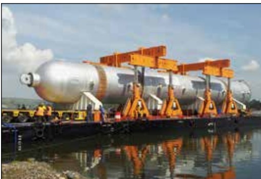
◀ Two SBL1100 gantry systems lifted the 1300 ton hydrocracker off the barge onto a SPMT Self-Propelled Modular Transporter.
